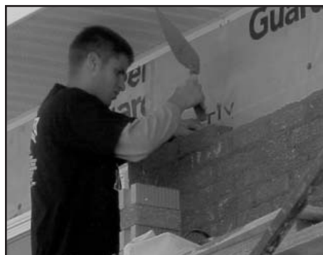
Dan Mau, a student at Southwest Wisconsin Technical College, from South Wayne, Wis., contributes his time and talents to the school's new student residence building.
