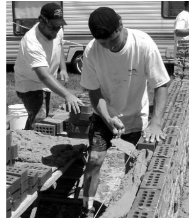
Winning mason Mike Boll shows skill and speed by laying an amazing 714 bricks in one hour.
