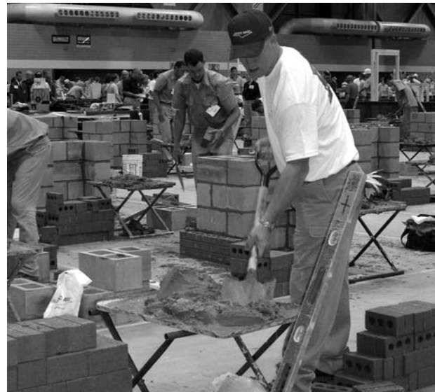
Mudslinger Ryan Nye, Pre Mix Industries, helps with providing mortar to the apprentices.
