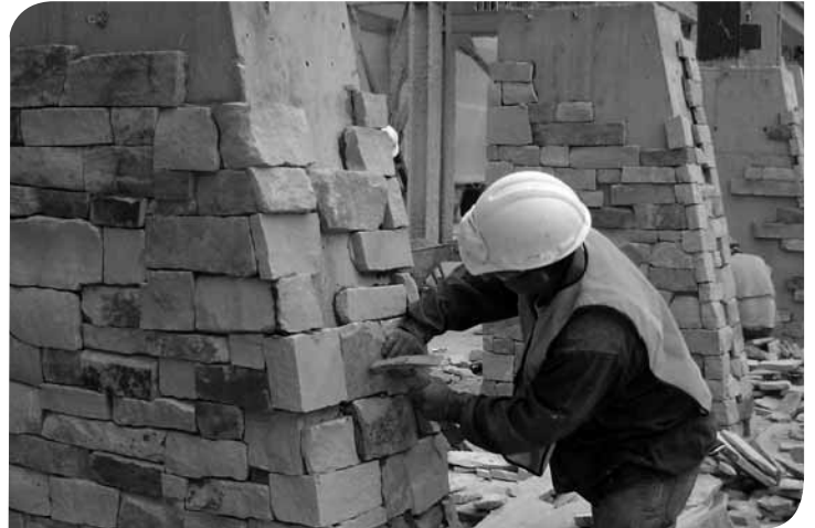
A Child Enterprises stone mason carefully fabricates the thin veneer into position without affecting the aesthetics of the stone. Several heavy thin veneer stones hang in the balance with the SPEC MIX PMSVM on the extraordinary piers that line the front of the hospital
