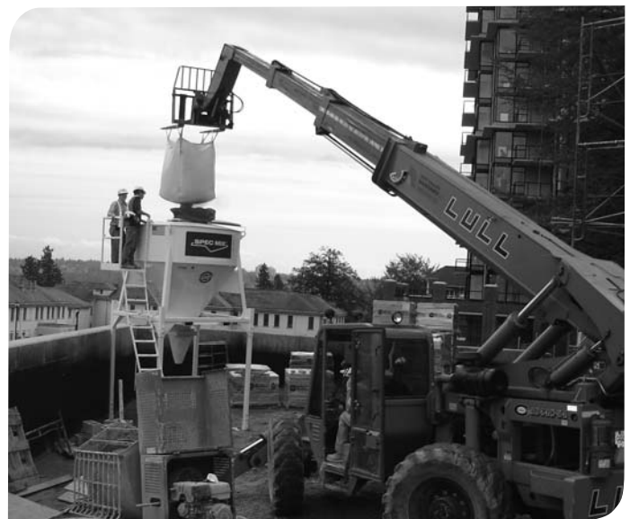
SPEC MIX/Target Staff show the Sun Valley Masonry crew the ease of loading a silo in New Westminster, BC.
