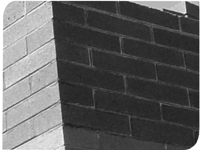
Photo #5: Photograph of a newly constructed wall with grouted cells. Note that the grouted cells were not covered. Shortly after a rain event efflorescence began to appear in the upper courses of the concrete masonry wall. This could have been prevented if the top of the wall was covered prior to exposure to rain.
