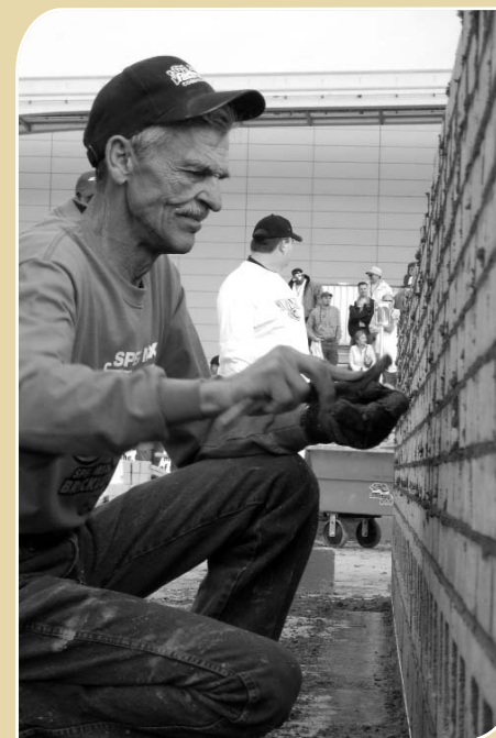
Bill Morrisette, from Morrisette Masonry, Chickamauga, GA, was the TOP CRAFTSMAN Award winner. Bill is seen here cleaning up his wall in the final seconds of the competition. He impressed everyone with his performance and the quality of his 603 brick wall.
