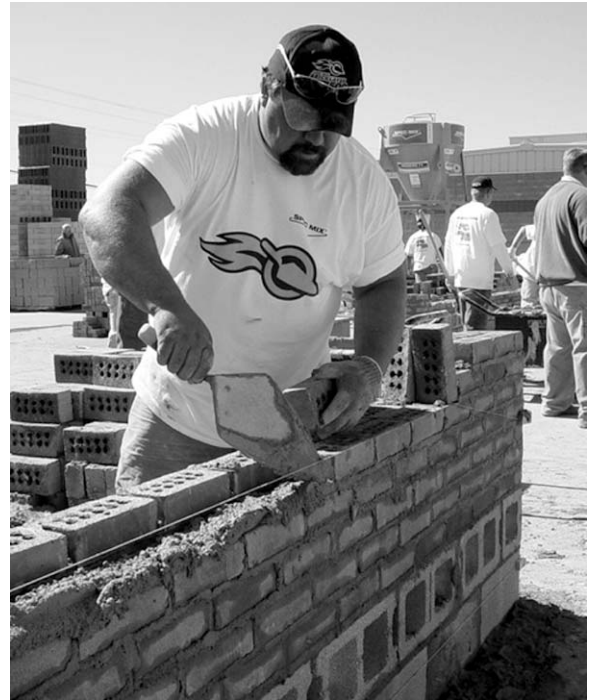
Tim Lowe works quickly and cleanly to win the Craftsmanship Award in the Michigan regional SPEC MIX Bricklayer 500, as well as take second place overall. The Craftsmanship Award was created in response to industry concern that not enough emphasis was being placed on quality of workmanship.
