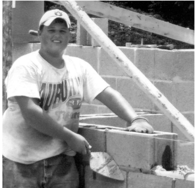
Josh Knudtson of Dawson, Iowa, checks his work during the 2003 National Masonry Contest held in conjunction with the SkillsUSA-VICA National Championships in Kansas City, Mo.
