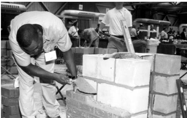
Errol McDonald lays another brick on his composite project in the post-secondary competition of the 2003 National Masonry Contest held in Kansas City, Mo., in conjunction with the Skills USA-VICA National Championships.
