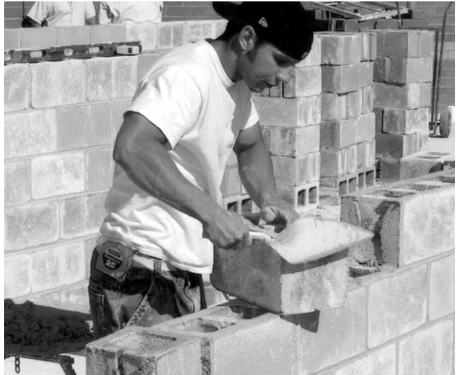
Joshua Garigali of Mesa, Ariz., builds a block wall. Garigali works as a journeyman mason for Sunnyside Masonry in Mesa, Ariz. Photo Credit: Scott Farence, f2pix, Inc.
